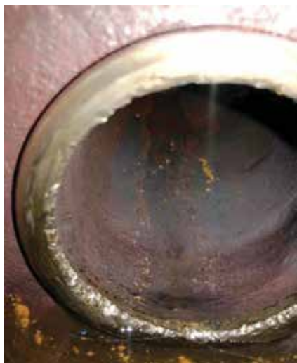
Figure 2: Seat damage caused by chattering
